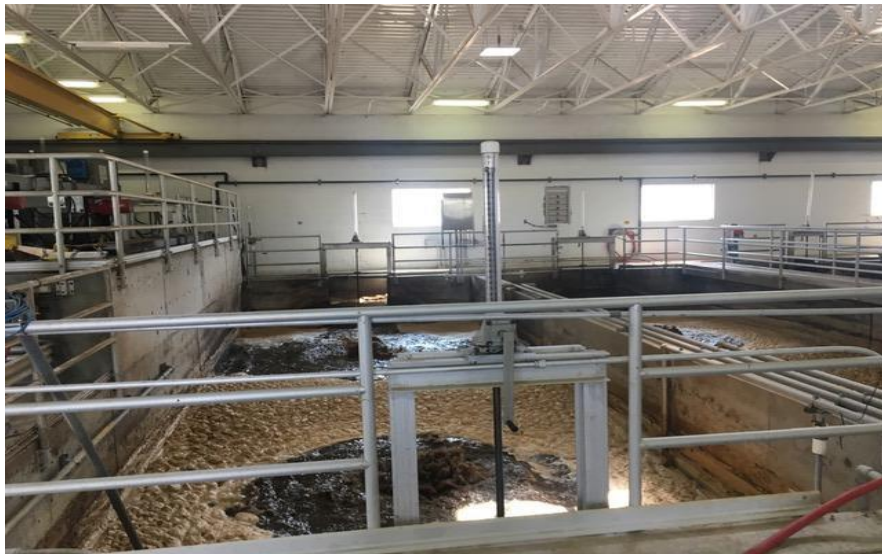
Fig. 5. The anoxic basins in the Hyrum WWTP.
